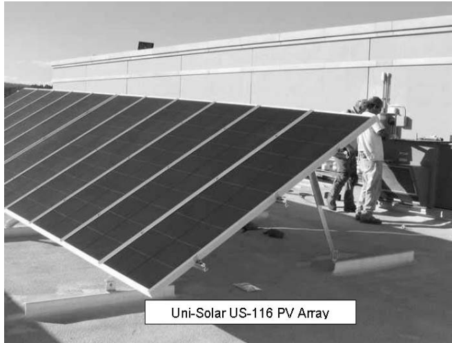
Figure 3 Santa Cruz Site: Uni-Solar's Framed Modules
